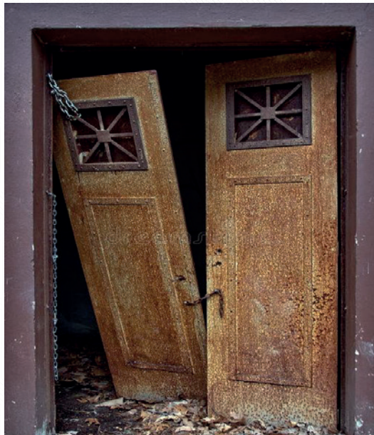
Figure 1 illustrates damaged external doors on the old library.
