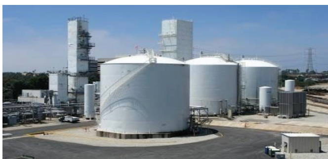
Figure 10.3: An air separation plant
